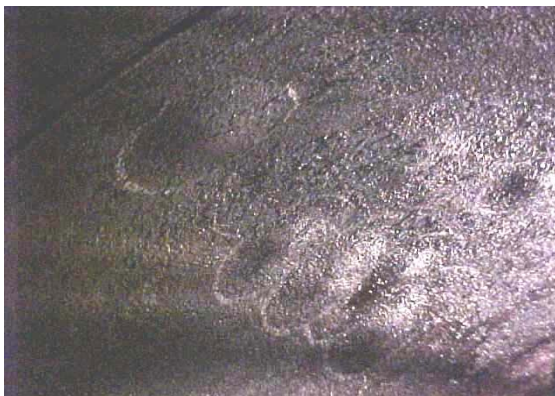
Photograph No.01: Series of blisters on the shell.
