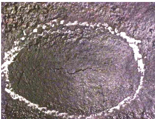
Photograph No.02: Close up view of a blister with branched cracks at its center.
