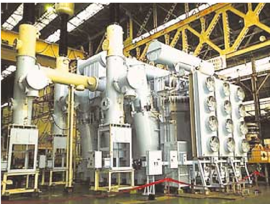
Fig. 1—View of Shop Test of 281.25-kV (525-kV) 1,060-MVA Double Rating Voltage Transformer. The shop test would be carried out by using test bushings, although the secondary side was connected with power cable. The test was first carried out in the 525-kV connection state and was repeated after changing to the 281.25-kV connection.
