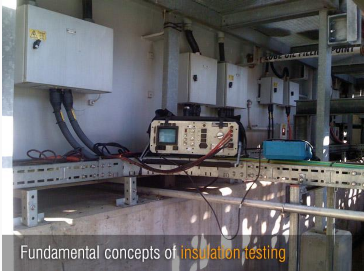
Fundamental concepts of insulation testing (on photo Digital Surge/ HiPot / Resistance Tester on site)
