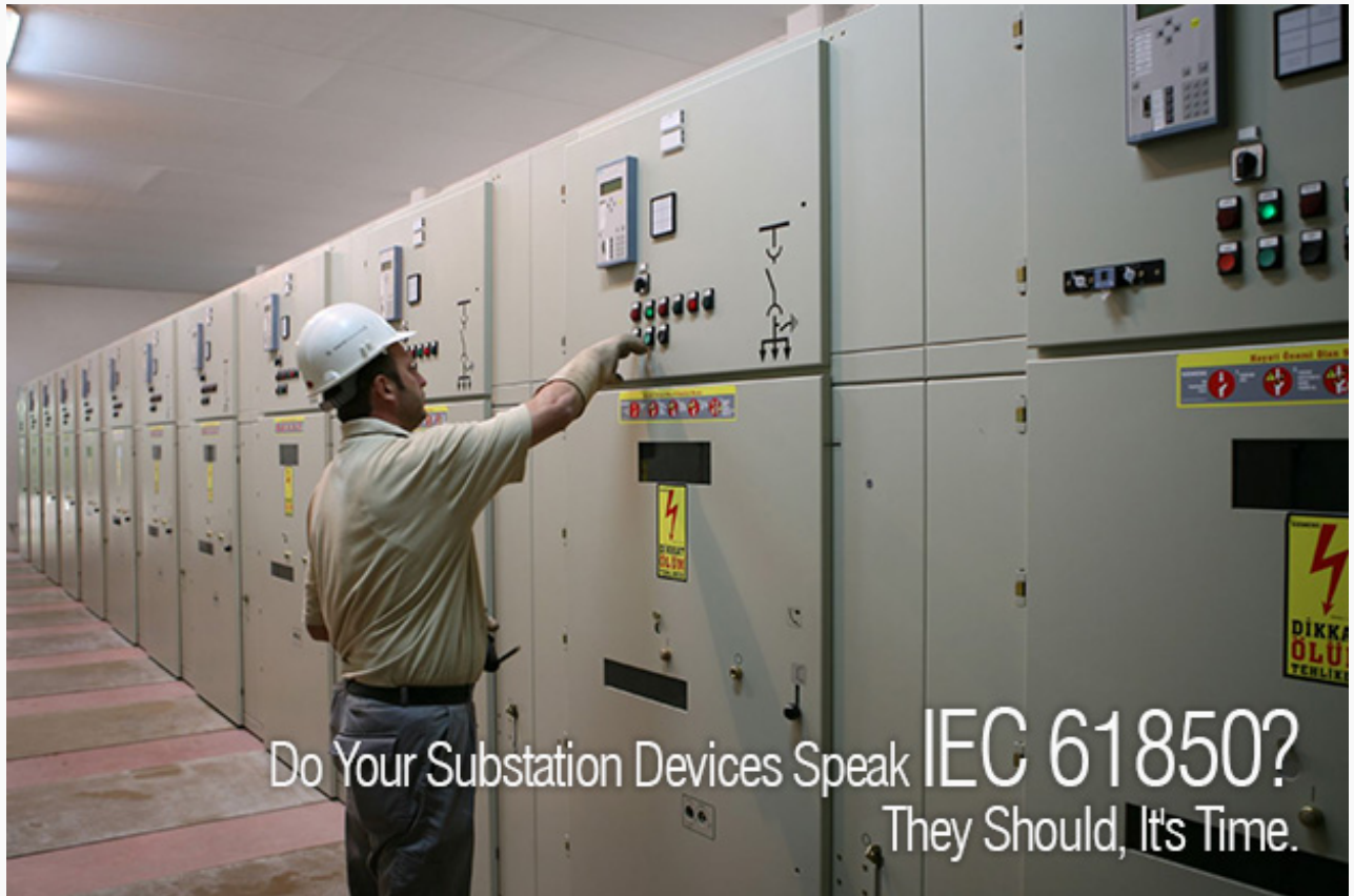
Do Your Substation Devices Speak IEC 61850? They Should, It's Time. (photo by Siemens A.Ş. - Siemens Türkiye)
