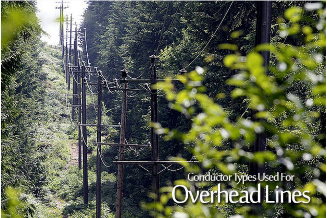
Conductor Types Used For Overhead Lines (on photo: Transmission Line 69KV Upper and 25KV Lower Near Cypress Area, Canada - by Wolf Read via Flickr)
