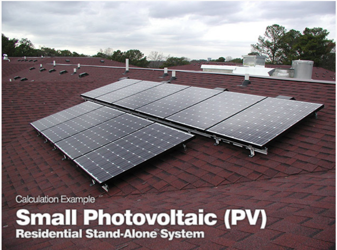
2kW Solar PV Array on Campus Crossings at Briarcliff (photo by Soenso Energy)
