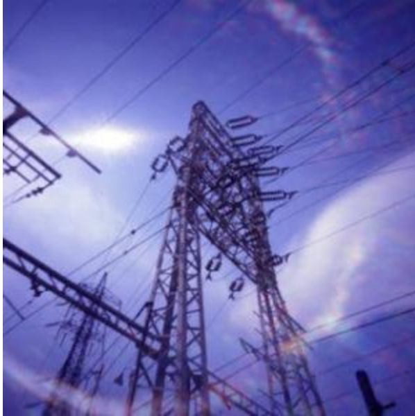
Ultimate distribution of Power after Generation
