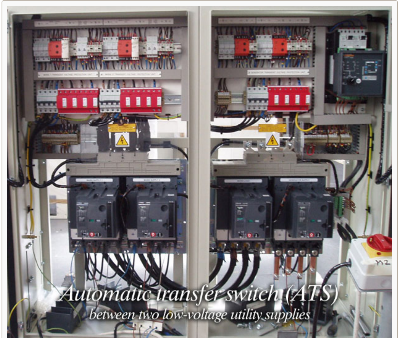
Automatic transfer switch between two low-voltage utility supplies (photo by Giffen Switchgear, UK)
