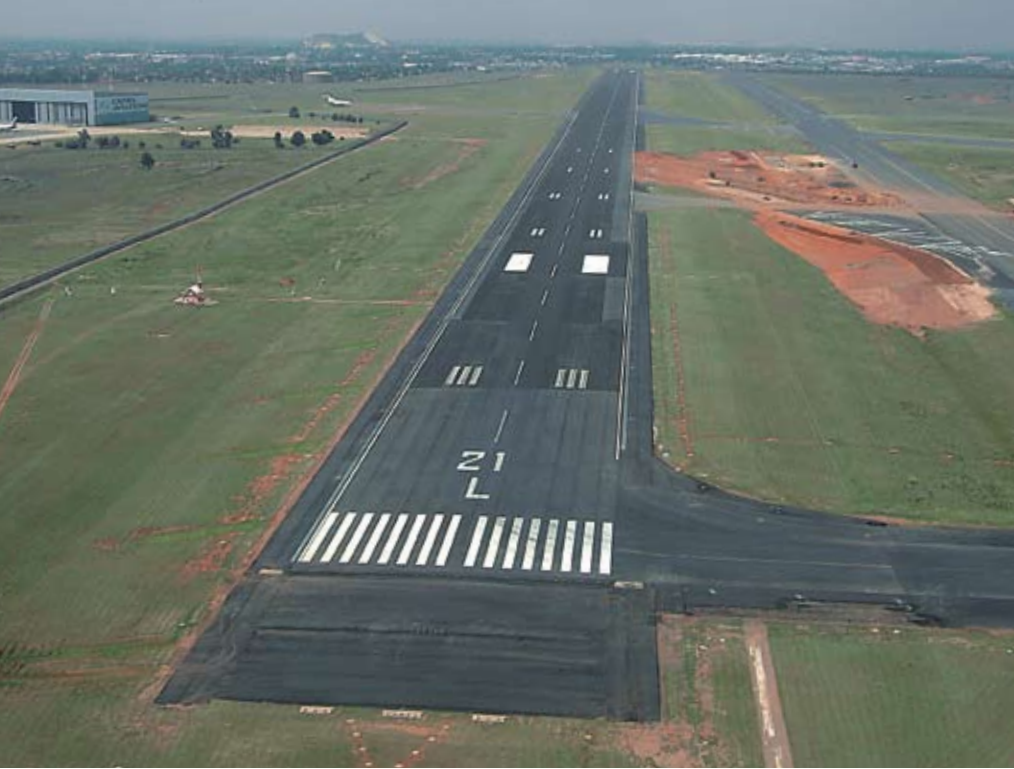
► An aerial view of the main runway with the Yankee taxiway on the right and a rapid exit taxiway being constructed
