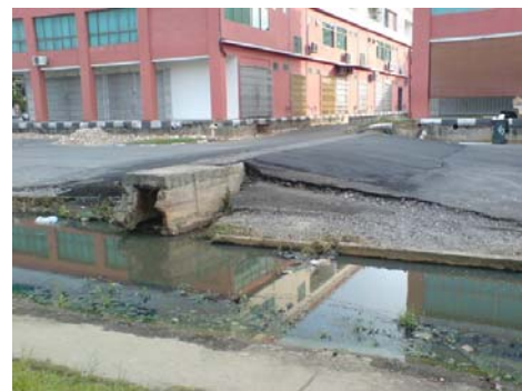
Fig. 2 Ground settlement caused poor drainage and road system in a commercial lot, Sibü.
