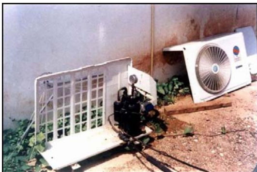
Fig. 3 Photograph of condensing unit of M-AC
