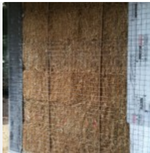
Bamboo is tied through the bales to lock them in place, courtesy of "Boa Constructor".
