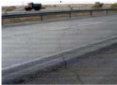
Fig. 5. Fissuring in Yazd-Maybod main road
