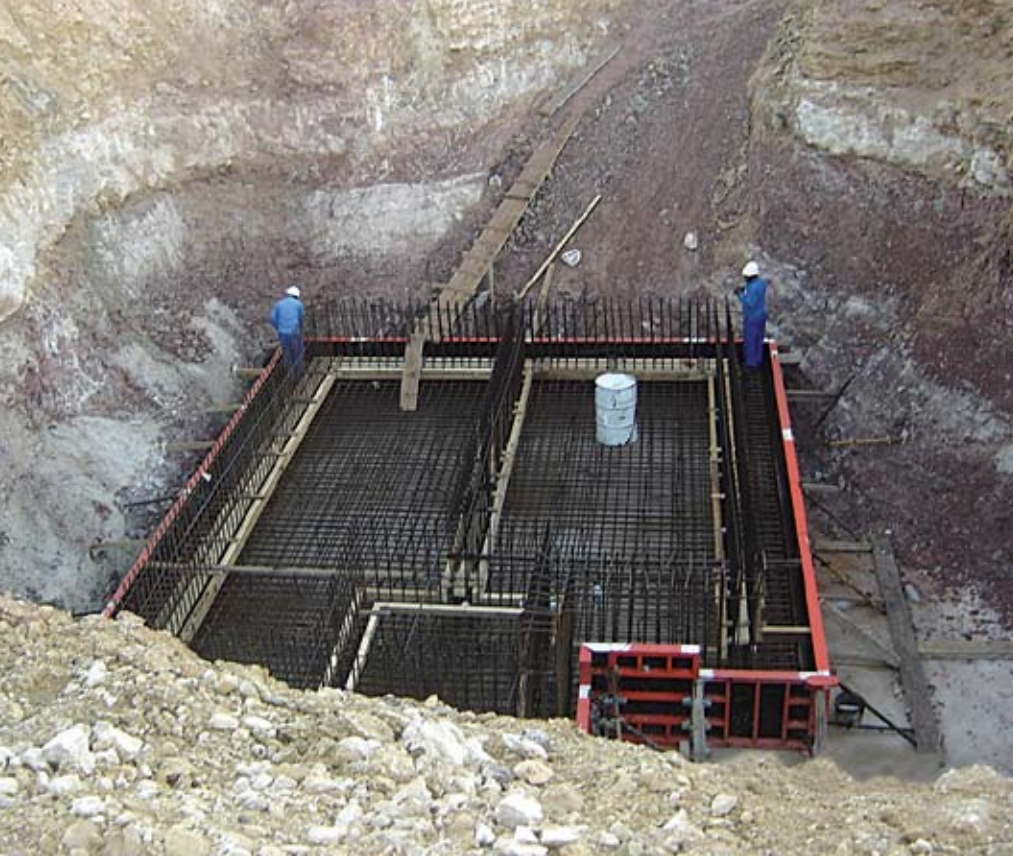
► Top left: Deep excavation for sewer pump station Above: Steel fixing for sewer pump station Bottom left: Earthworks with pond B1 in background
