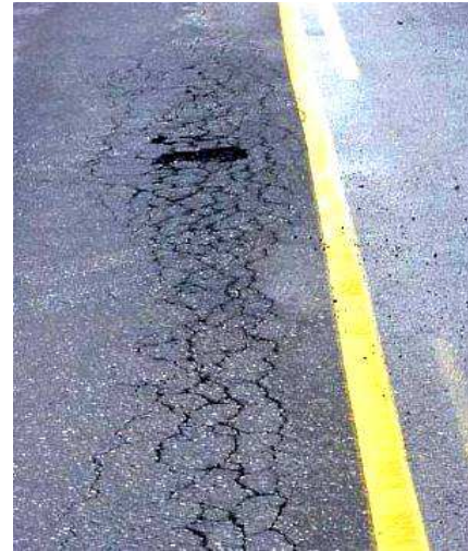
Fig. 4 fatigue causes pothole
