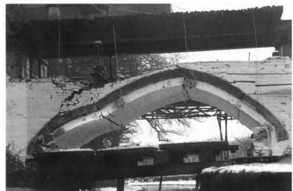
Figure 6: Collapse of the Bridgemill arch bridge. (Source: http://archive.niees.ac.uk/talks/dem/nenad_bicanic.ppt )
