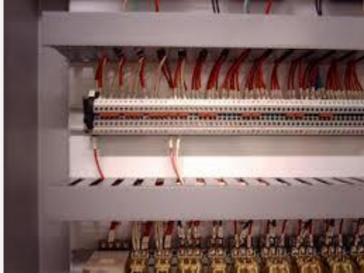
Example of good spacing between the terminals and the wireway.
