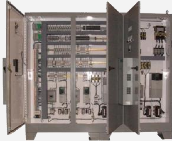
Large Control Panel Wiring Example. What are some good practices? What could be improved? Click to enlarge
