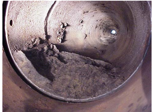
FIGURE 2. Contamination Buildup at the Plate Seat of an Orifice Flow Meter
