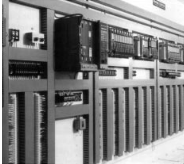
Figure 3. Placement of PLC components.
