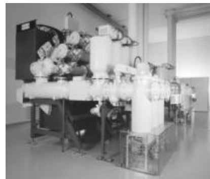
Fig. 1: 145 kV GIS substation with advanced design
