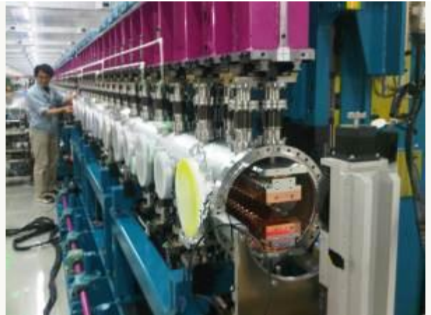
The undulators are being installed. The narrow stripe inside the tube, flanked by magnets, is where the electrons are sent on their wiggling path. During operation this tube is under vacuum.
