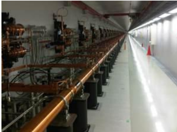
The long accelerator line. electrons are accelerated over a distance of more than 400 meters. Once accelerated the electrons are fed into the undulators.
