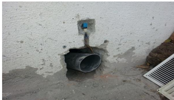
Opening in the wall with extraction tube and humidity sensor (blue)
