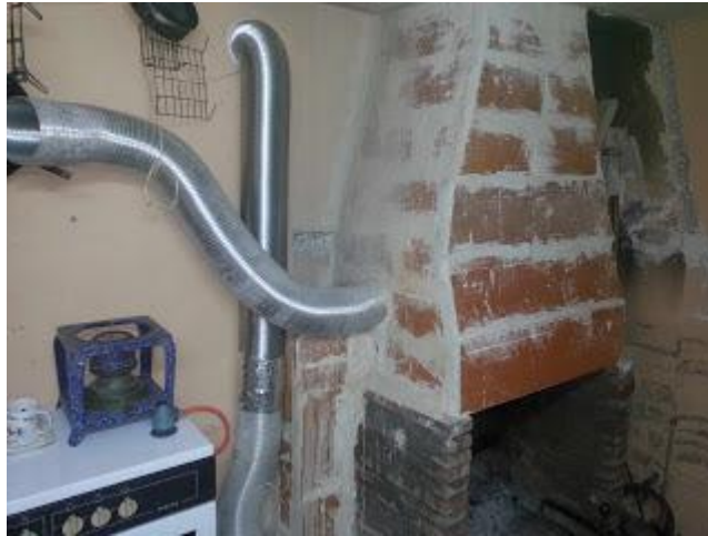
Low heat with heat removal by natural draft failing to place the drywall
