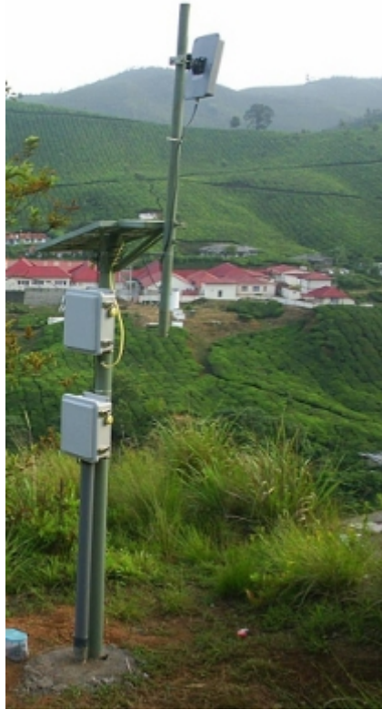
Fig. 8. C3 Sensor Column of Main Deployment
