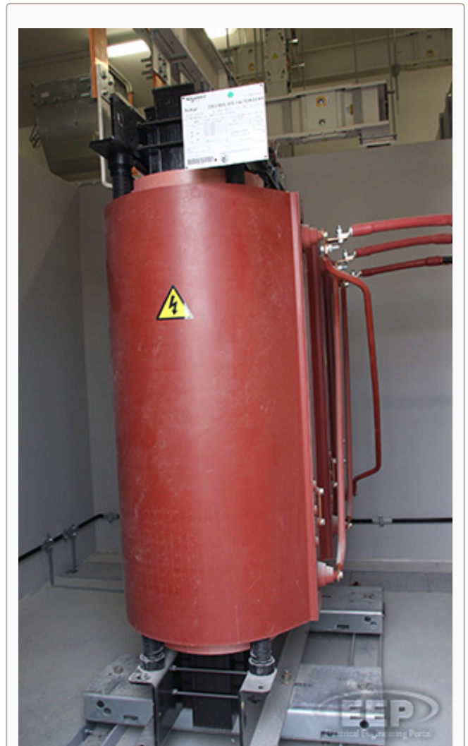
Trihal - Dry-type transformer 1600 kVA 10/0,42kV connected to busbar system Canalis KTA 2500A (Schneider Electric)
