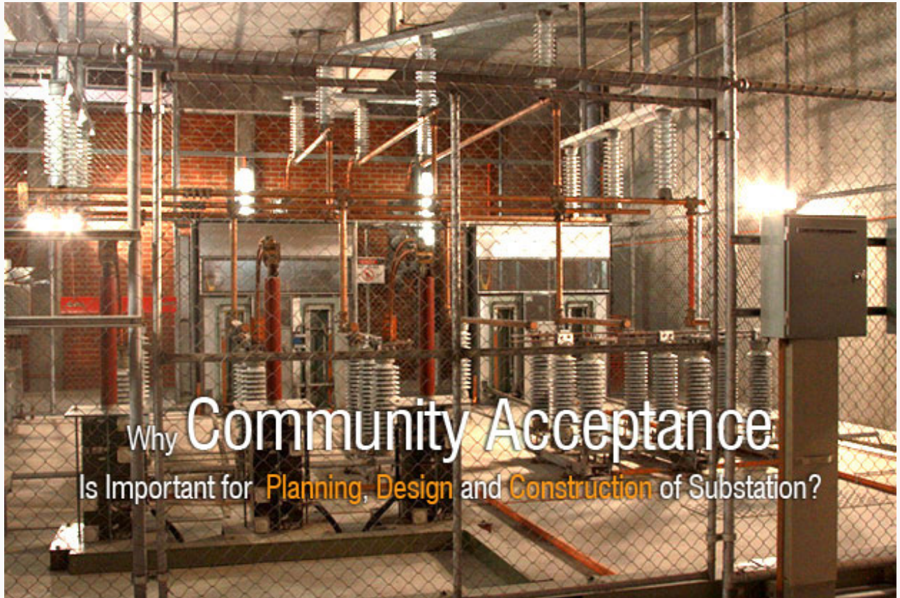
Power Substation that converts electricity from 66kV down to 11kV (photo by Marcus Wong via Flickr)
