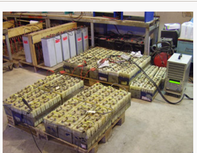
NiCad Batteries being charged
