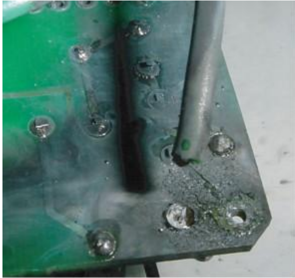
Figure 7. Example of dielectric breakdown between line traces on a printed circuit board used in an EMI filter and a grounded surface (filter shield).
