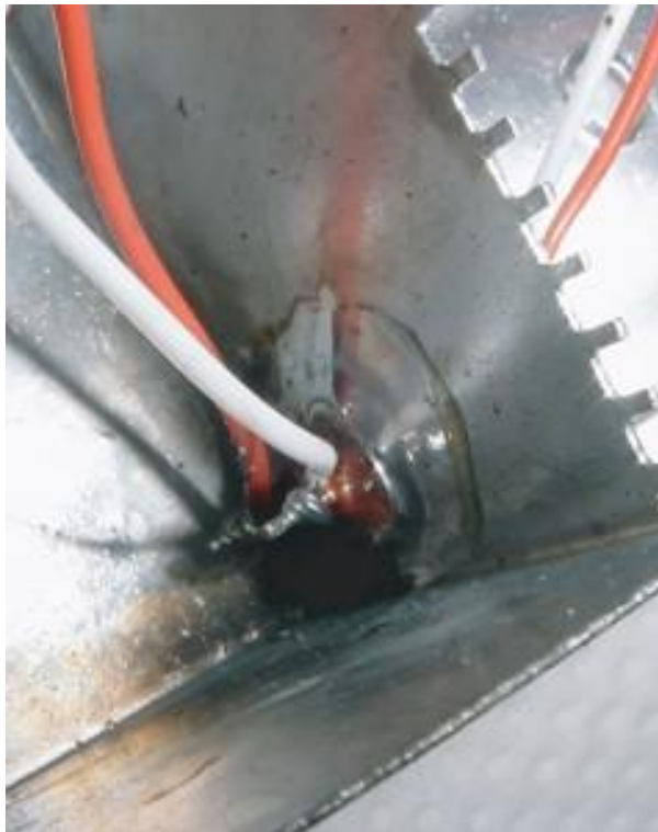
Figure 3. Example of a Y capacitor failure in shielded EMI filter.
