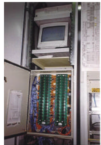
Fig 3: Central Marshalling and Control PC
