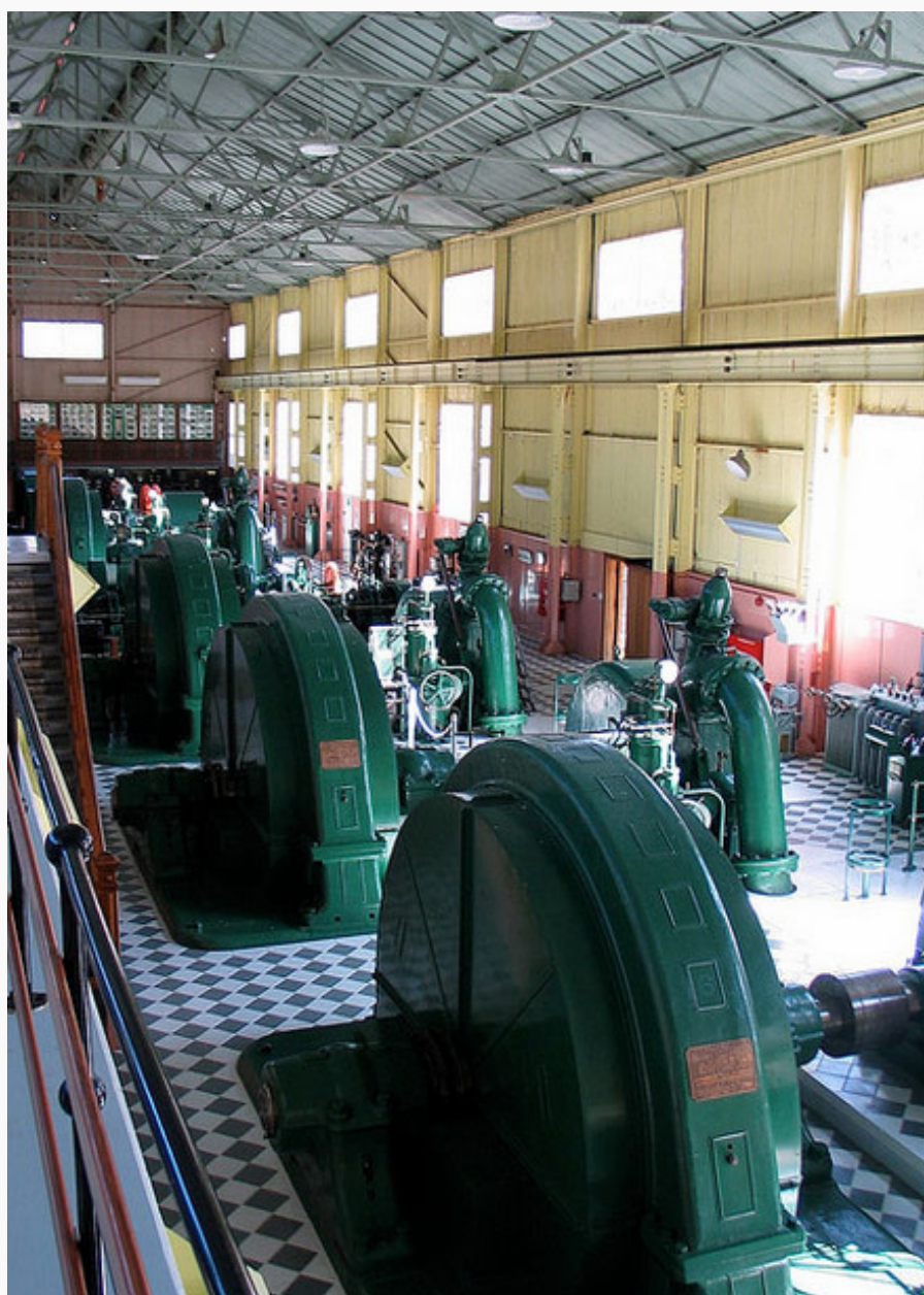
Waddamana Power Station A generator room (photo by Ben Short via Flickr)
