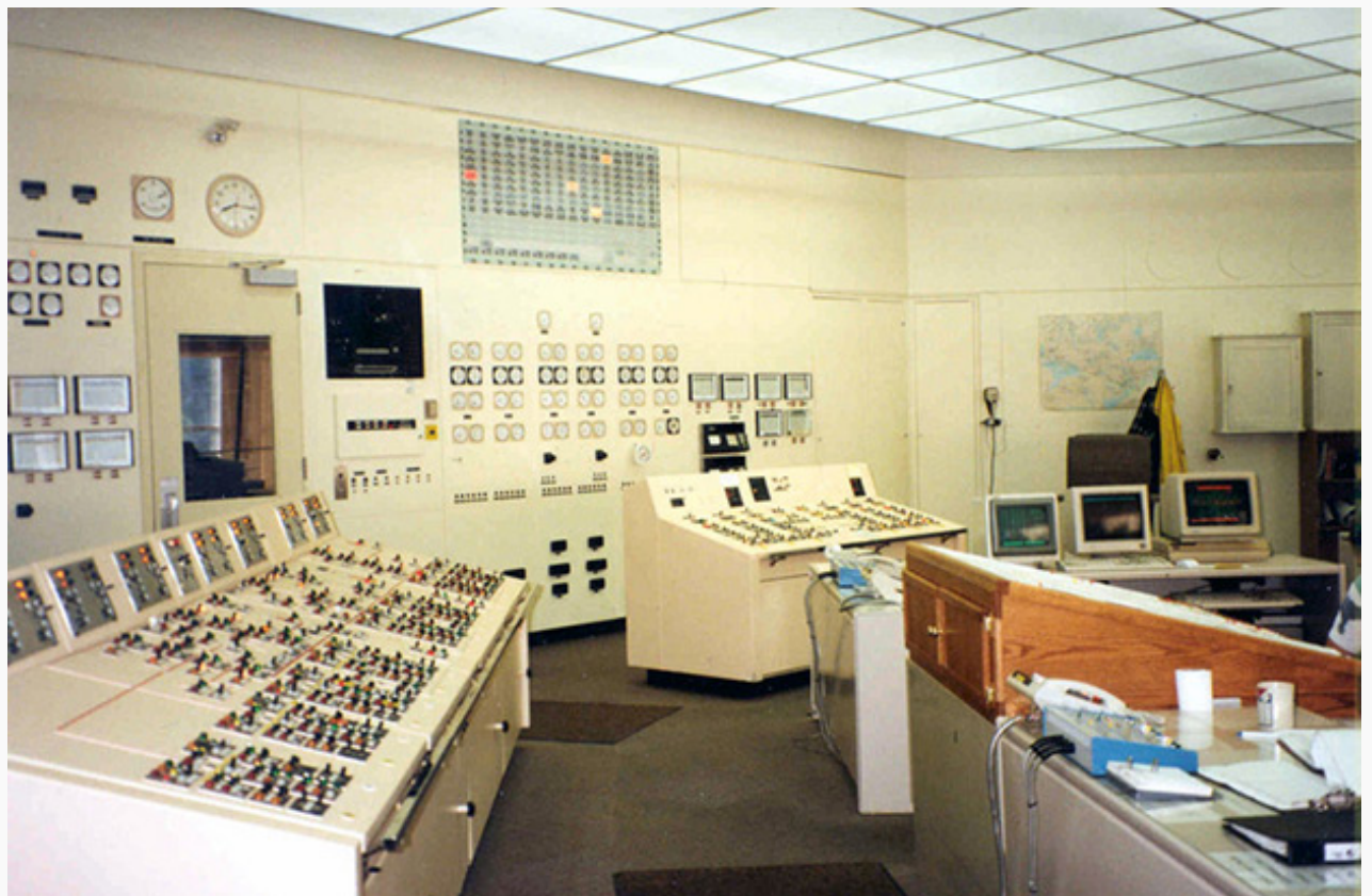
Ontario Hydro Niagara Falls Power Plant Control Room
