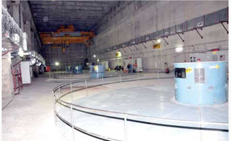
Elevation of the crane rail in hydropower plant
