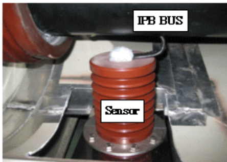
Fig. 6. Ceramic sensor installed into a generator's IPB
