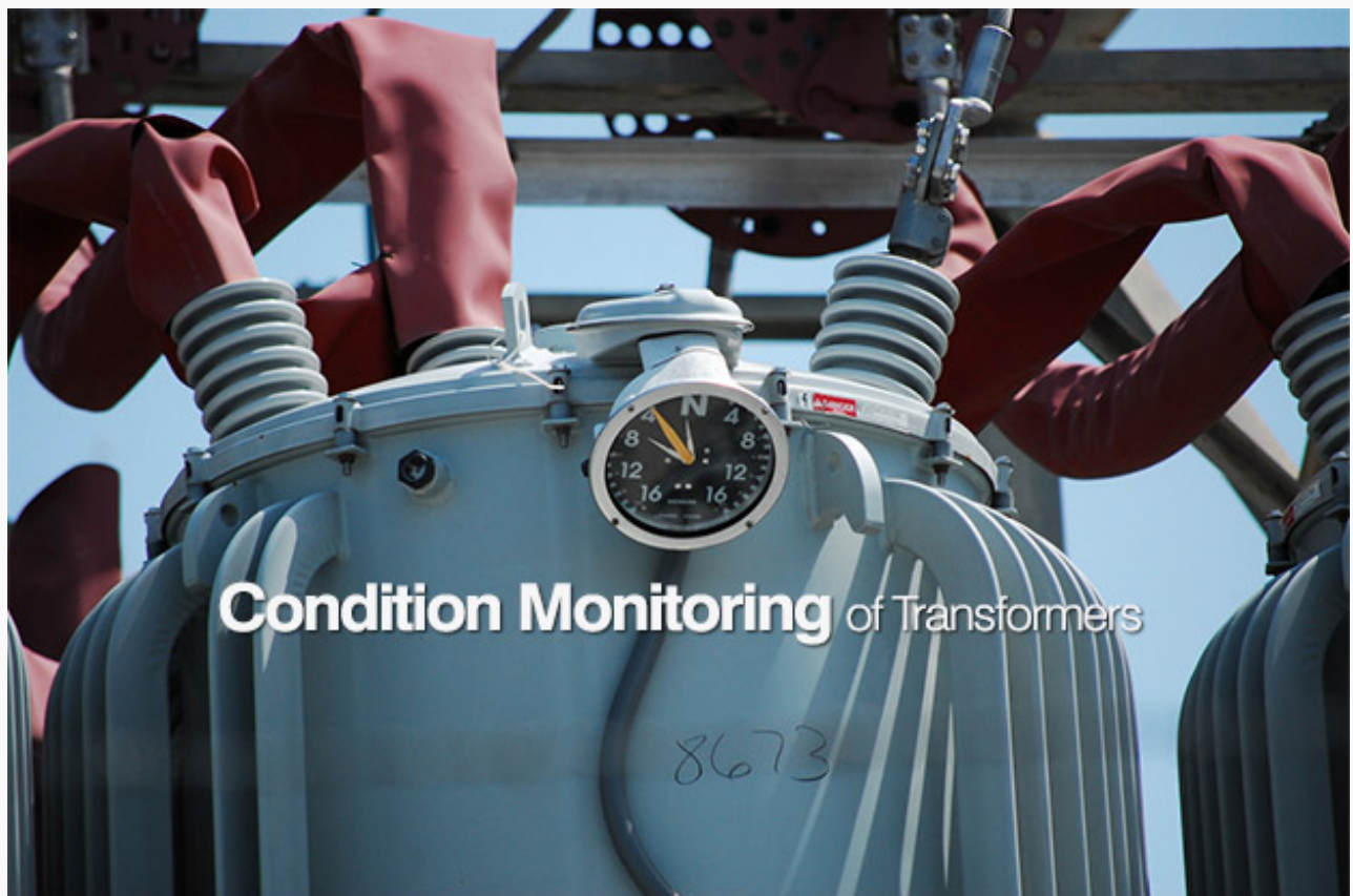
Condition Monitoring of Transformers (on photo: distributive transformer; by Gazoogleheimer via Flickr )
