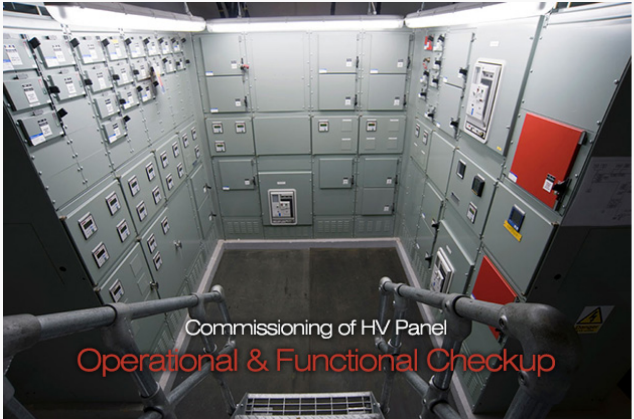
Commissioning of HV Panel - Operational and Functional Checkup (on photo Macmillan – New High Voltage Panel by Skilz Building Solutions)
