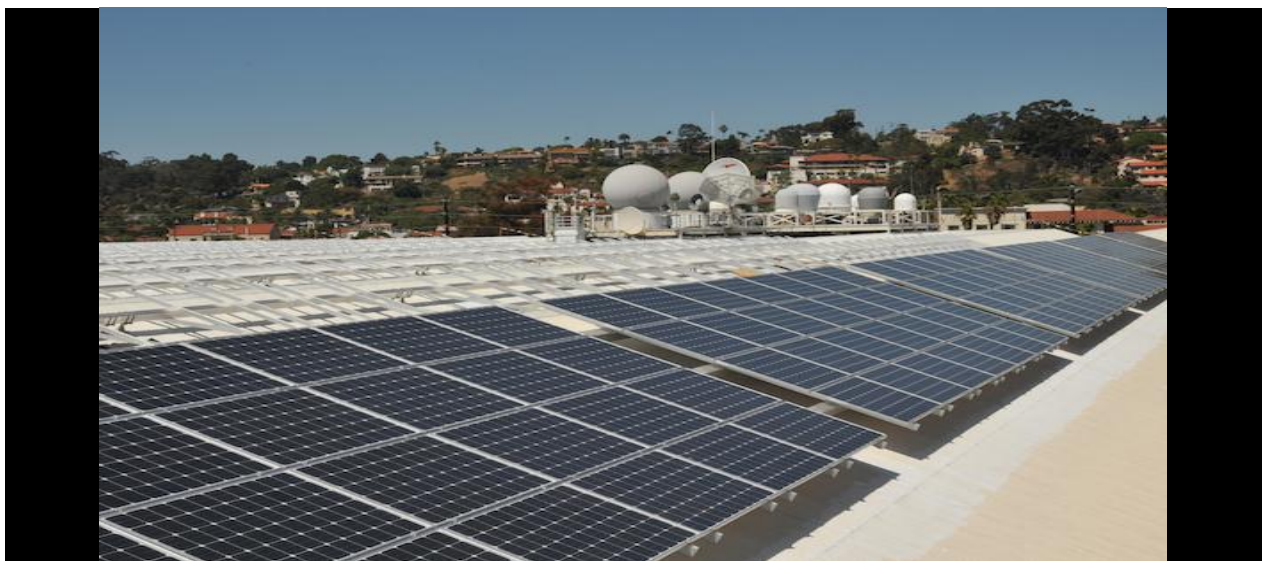
Solar panels at Space and Naval Warfare Systems Command Headquarters (U.S. Navy photo by Rick Naystatt).
