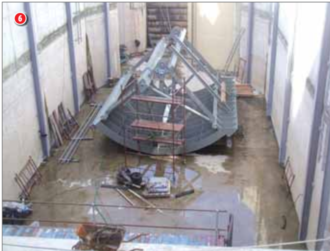
6 Assembling of the lock gates 7 and 8 and 9 and 10 Views of the completed canal boat lock
