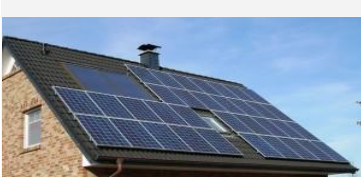
Solar Panels on a Roof by Pujanak (click picture for source)
