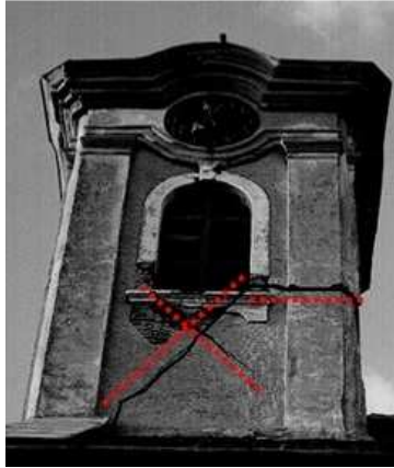
Fig. 15 Cracks at bell tower
