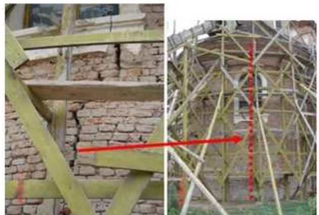
Fig. 14 Cracks at the eastern wall
