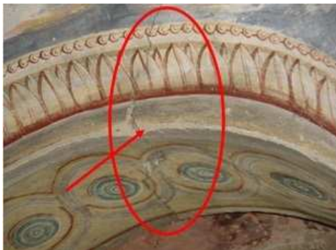
Fig. 16 Cracks at arches
