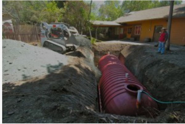
Rainwater cachment tank
