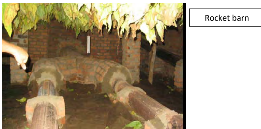
Fig 3: Rocket Barn Heat Exchanger
