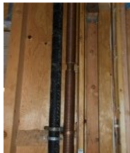
Shower Heat Recovery
