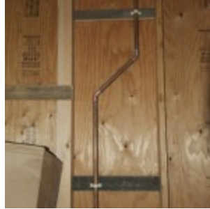
1" Copper Pipe in the Wine "Cellar"
