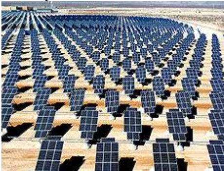
Photovoltaic solar array at Nellis Air Force Base, California. Source: U.S. Air Force
