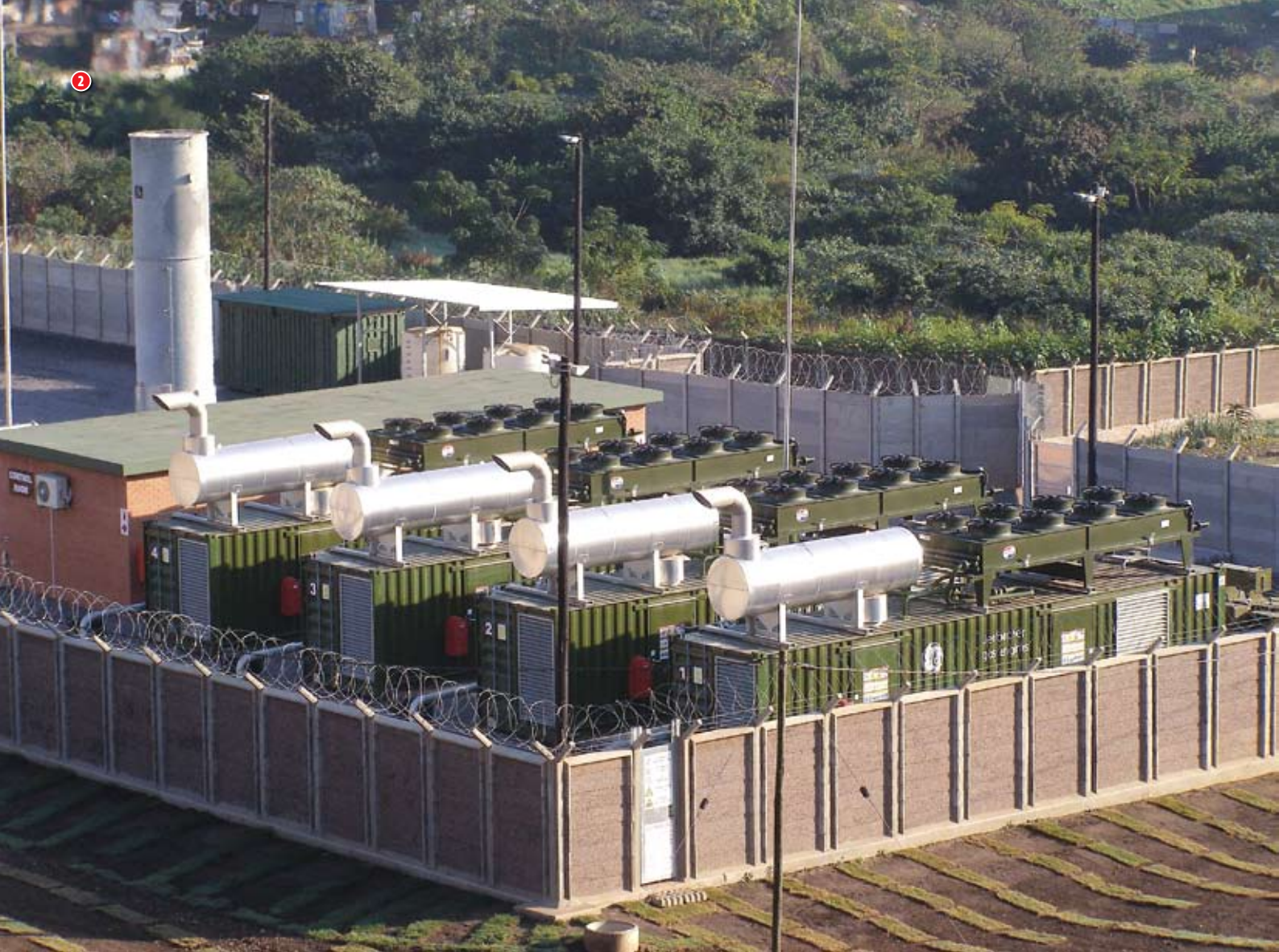
2 Landfill gas recovery – power generation units, Bisasar Road, Durban
