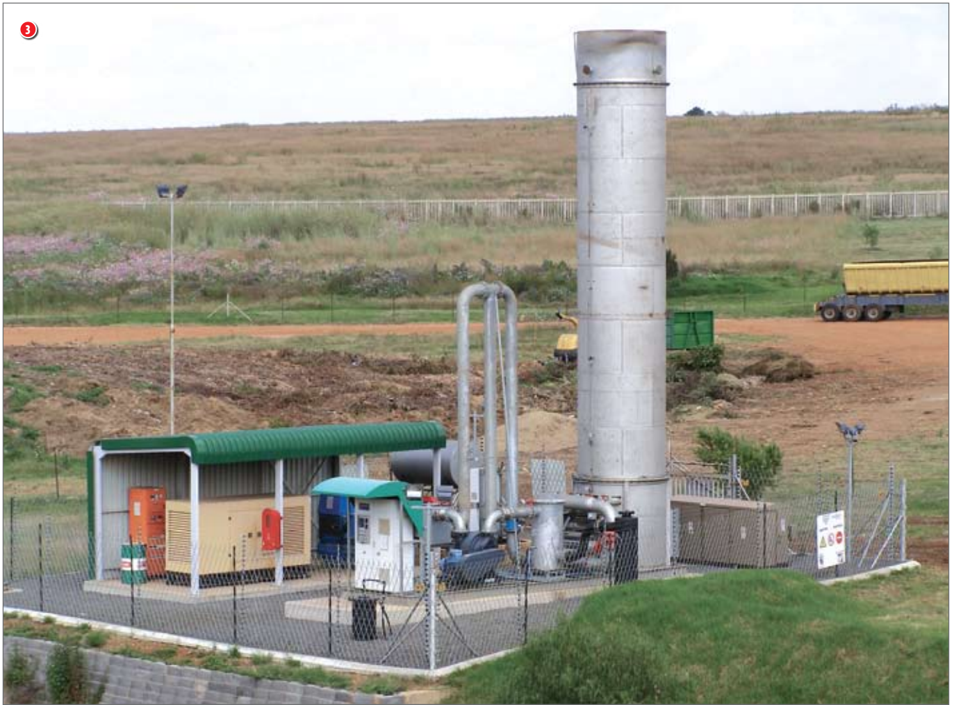
3 The 3 000 Nm 3 /h flare at Rooikraal landfill, Ekurhuleni Metro
