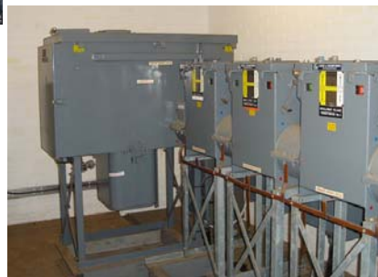
Typical indoor distribution substation
